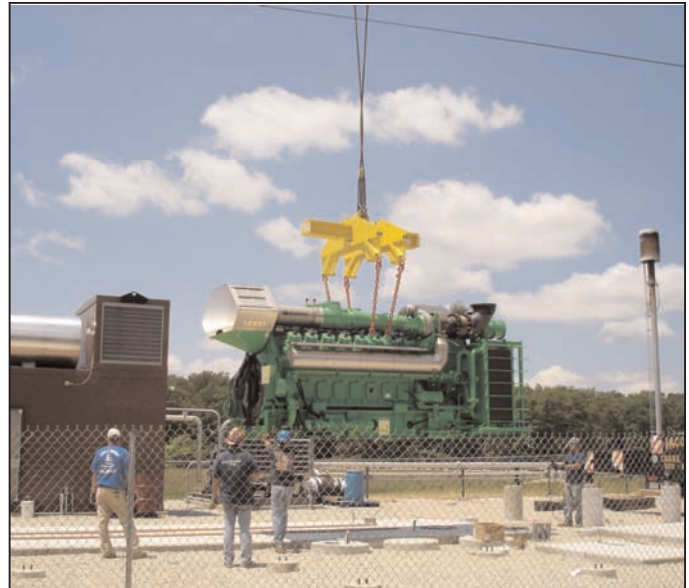
The second generator began operating in August 2006.
