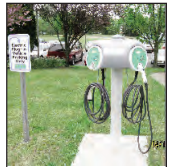
ACUA's AeroVironment charging stations at the Haneman Environmental Park.
